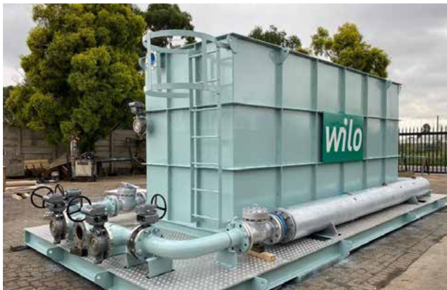
One of the holding tanks, which is used on the 950 and 450 metre mark Source: Wilo SE
